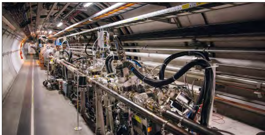
Excavating odderons Part of the TOTEM installation in the LHC tunnel 220 m downstream from the CMS experiment.
