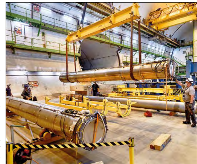
Dump upgrades Upgraded LHC external dumps with new instrumentation, beam windows and support systems being fitted into their new frames, ready for installation.
